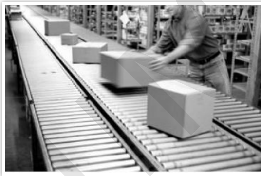
FIGURE 11: Motorised Roller Conveyor
